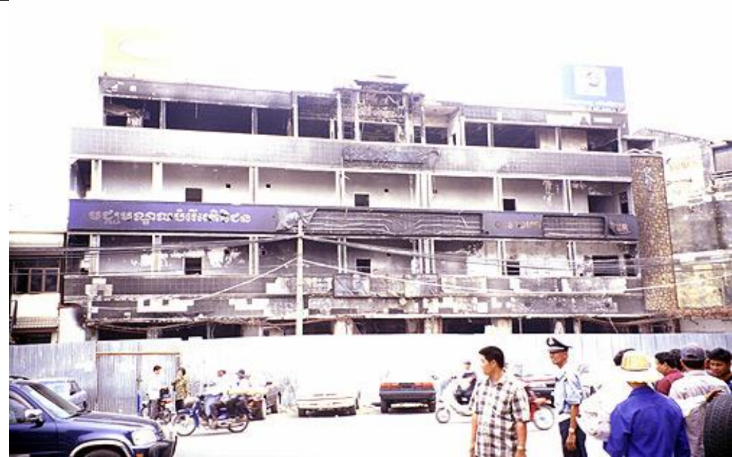
The offices of Cambodia Shinawatra Telecommunications, firebombed, windows smashed, with masonry damage.
